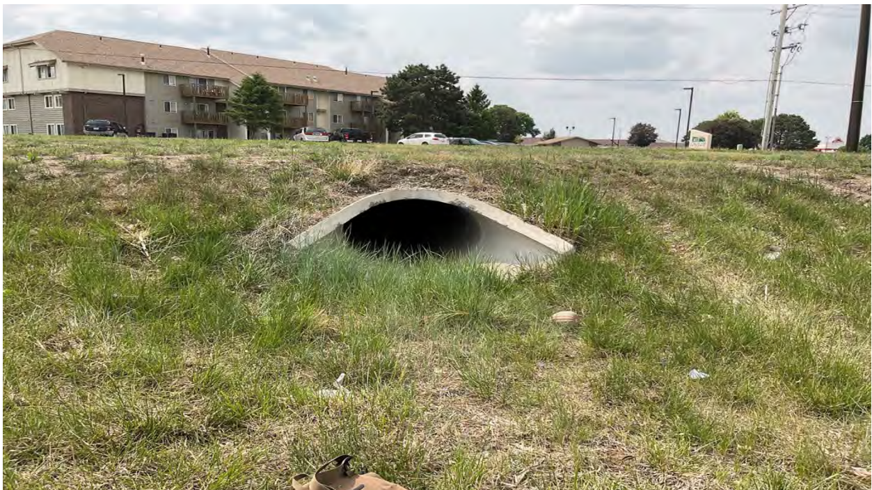
Photo 6 – View looking south from the north side of W Capital Avenue. Photo depicts a culvert structure under W Capital Avenue.
